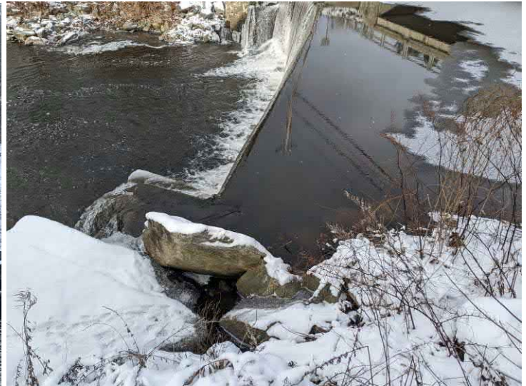
November 2021 – Flow through left abutment
